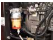
Diesel Filter with water separator
