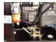
Coolant preheating and air preheating
